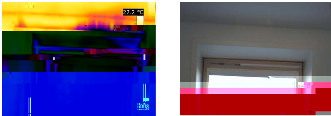
Figure 5. Infrared and normal picture of north-west facing window taken during blower door test.
